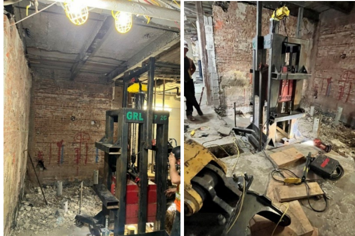
Figures 14 and 15. Dynamic load testing frame with elevator shaft footprint in background.
